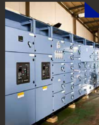
LV DISTRIBUTION BOARDS
